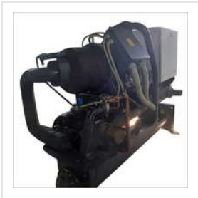
Commercial Chillers Plant
