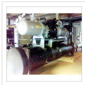
Commercial AC Plant Maintenance Services
