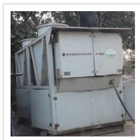
Air Cooled Chiller Plant Maintenance Services
